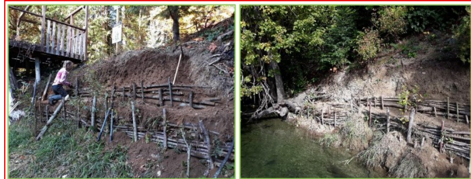
Figure 7. Construction of a live-stake wattle fence at two CSSP 2018 sites along Cowichan River
